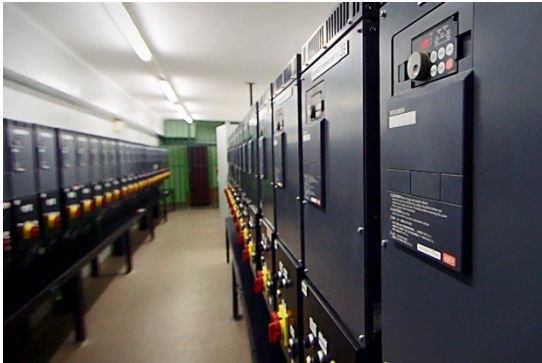
Picture 2: Special software was developed for inverters to meet the requirements of mixing of control modes (between fully automated and manual) and synchronisation of many drives in optical fibre communications.
